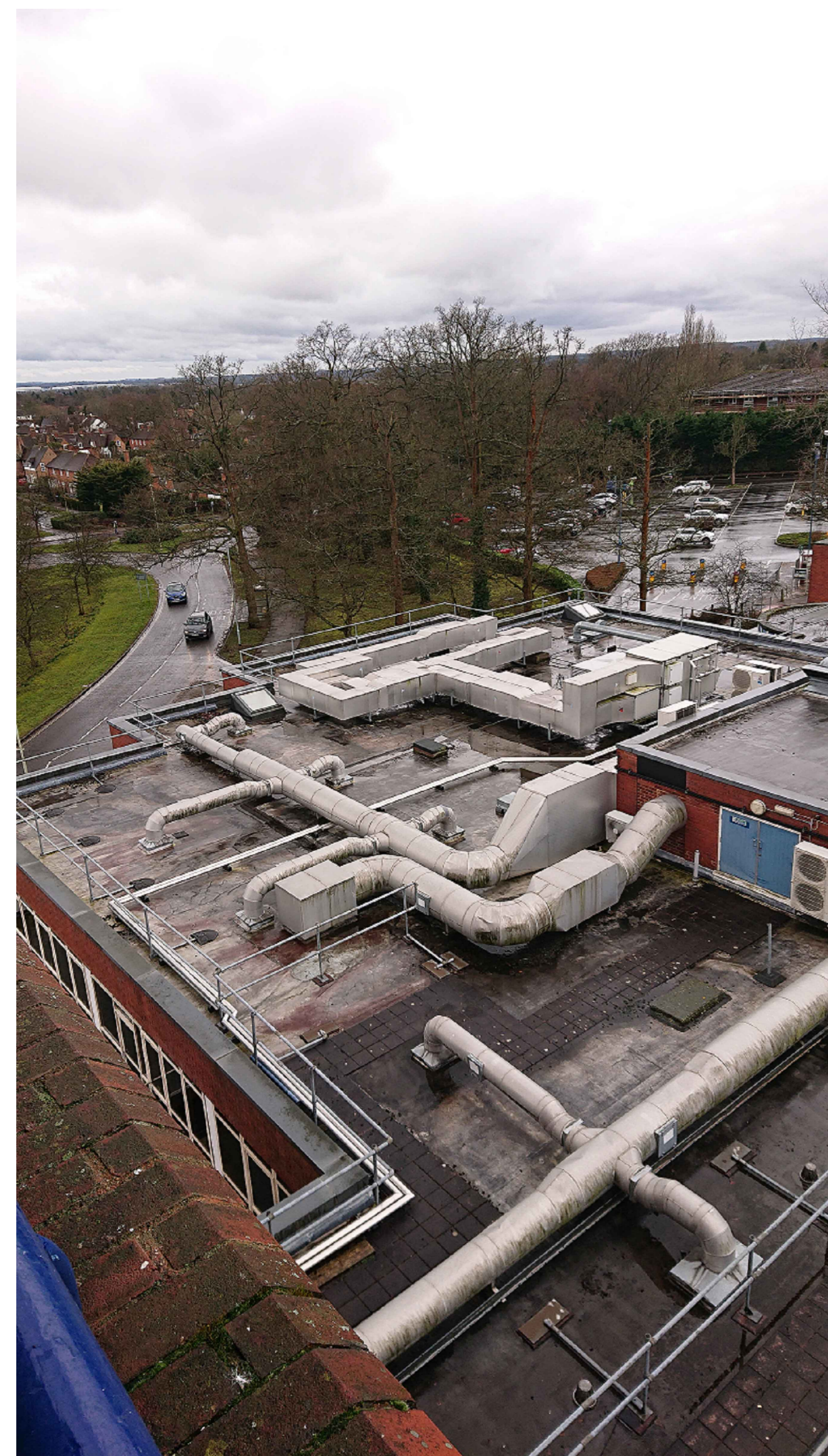
EXISTING ROOF MOUNTED PLANT AND EQUIPMENT
