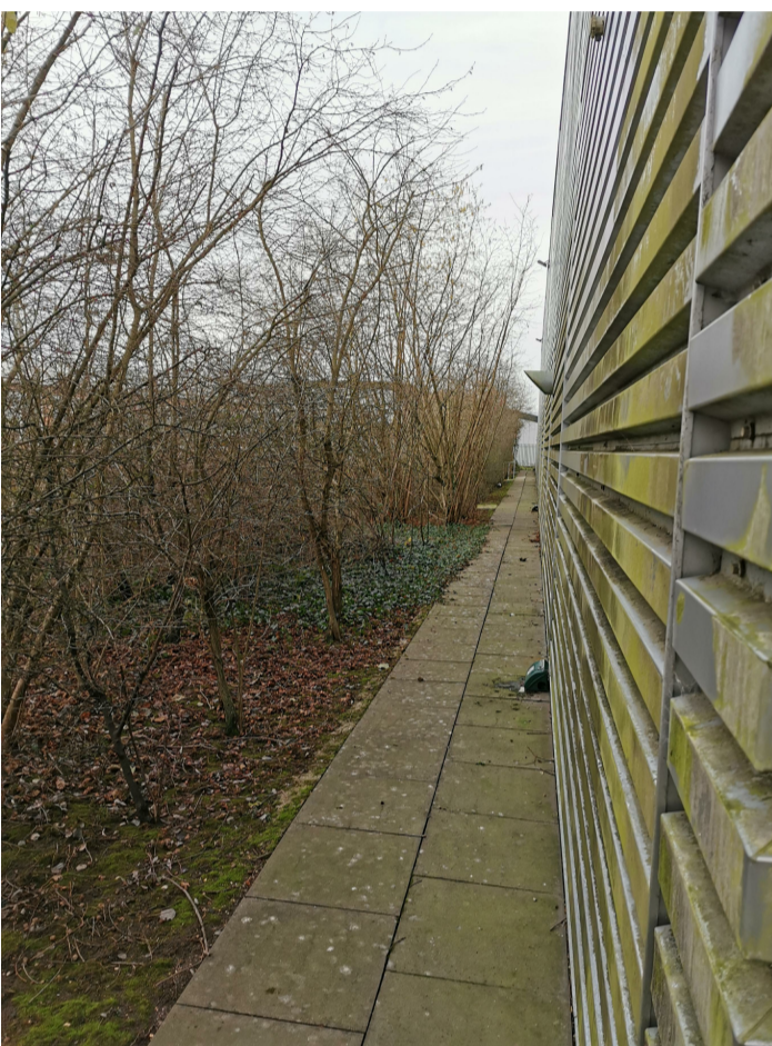
2 View from side of the building where new fire escape is being installed
