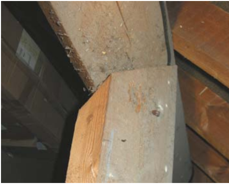
Photograph 11: Bat dropping on timber
