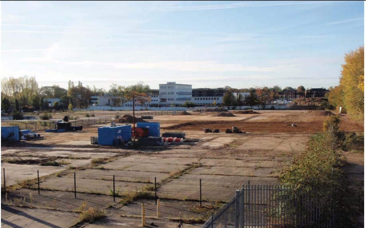
Former Polycell factory area following removal of groundwater treatment system and backfilling of the tank farm excavation.
