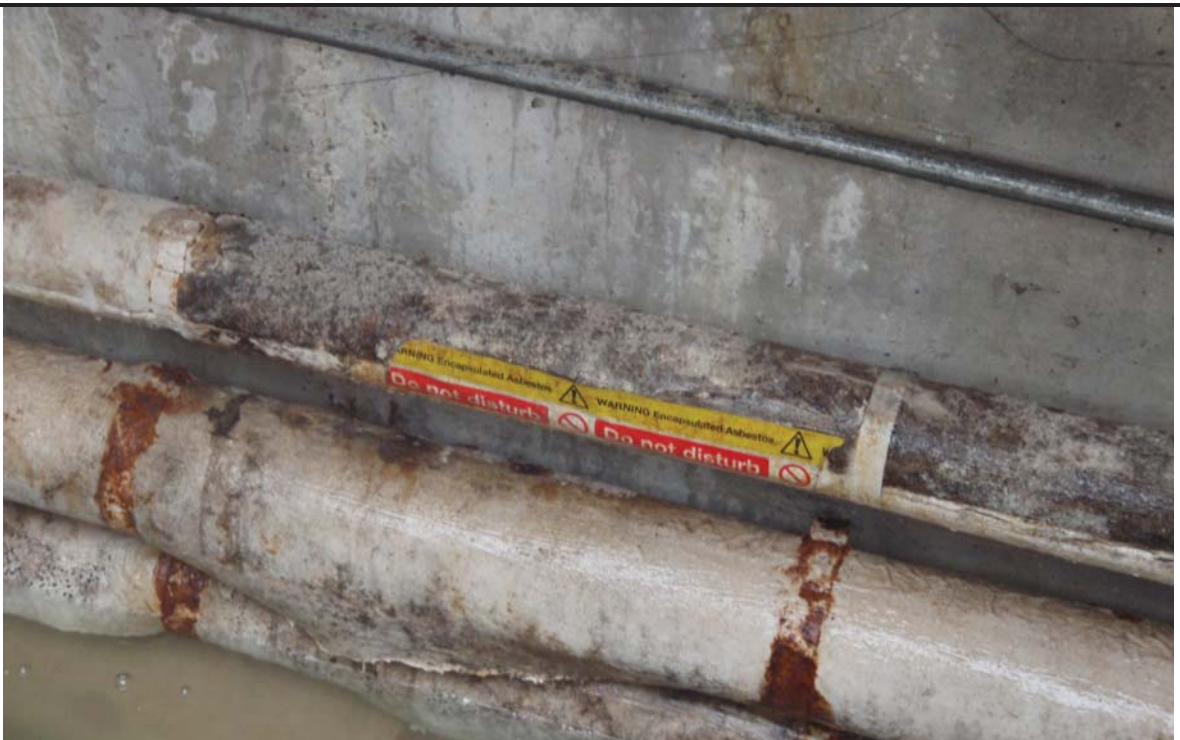
Lagged pipe and asbestos warning signage in water filled service duct in the south of the Site.
