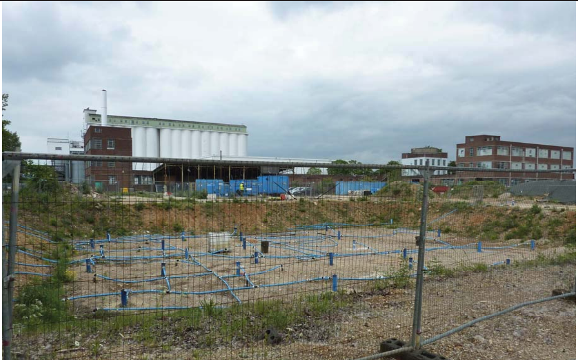
Polycell factory tank farm area – groundwater treatment system in operation following removal of tanks and impacted soils.
