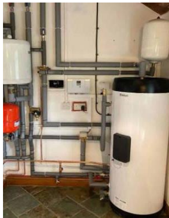
Services: Air Source Heat Pump
