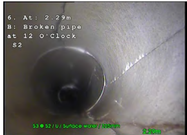
Photo: 47_47_579_A.jpg, 00:00:30 2.29m, Broken pipe, from 12 to 12 o'clock, Start
