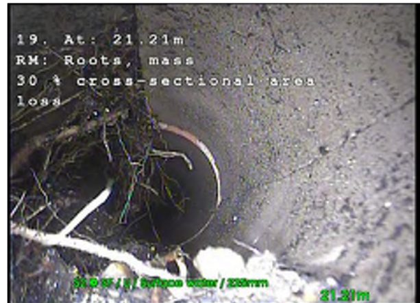
Photo: 42_42_364_A.jpg, 00:03:28 21.21m, Roots, mass 30 % cross-sectional area loss
