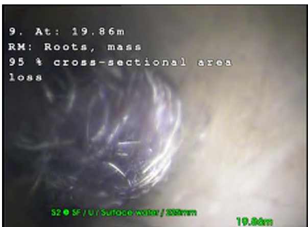
Photo: 39_39_327_A.jpg, 00:01:34 19.86m, Roots, mass 95 % cross-sectional area loss
