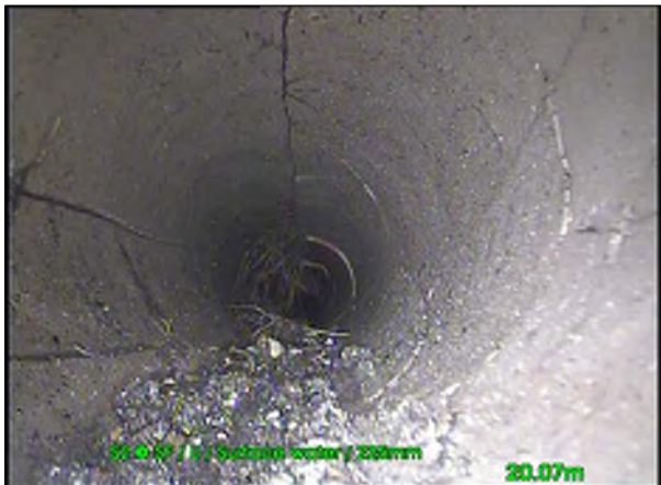
Photo: 42_42_363_A.jpg, 00:03:12 20.09m, Fracture, multiple, from 12 to 12 o'clock, Start
