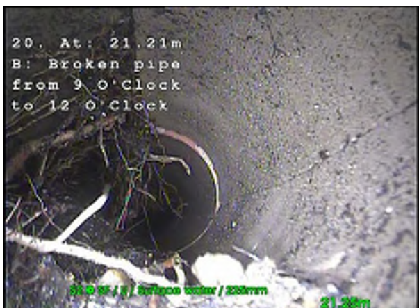
Photo: 42_42_365_A.jpg, 00:03:31 21.21m, Broken pipe from 9 O'Clock to 12 O'Clock
