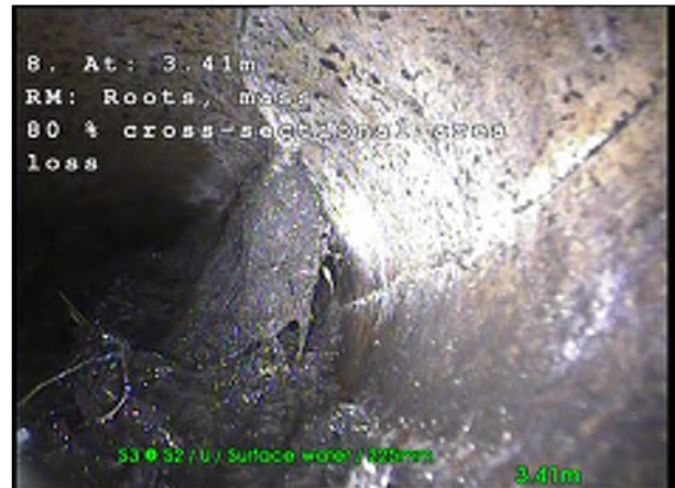
Photo: 45_45_399_A.jpg, 00:00:34 3.41m, Roots, mass 80 % cross-sectional area loss
