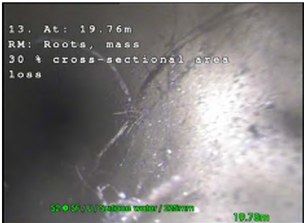
Photo: 41_41_342_A.jpg, 00:02:59 19.76m, Roots, mass 30 % cross-sectional area loss
