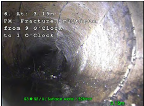
Photo: 45_45_397_A.jpg, 00:00:29 3.15m, Fracture, multiple, from 9 to 3 o'clock
