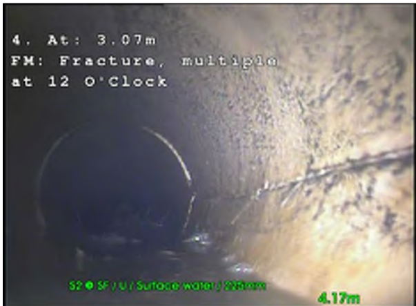
Photo: 39_39_322_A.jpg, 00:00:16 3.07m, Fracture, multiple, from 12 to 12 o'clock, Start
