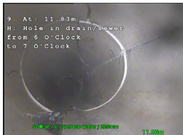
Photo: 41_41_338_A.jpg, 00:01:36 11.83m, Hole in drain/sewer from 6 O'Clock to 7 O'Clock
