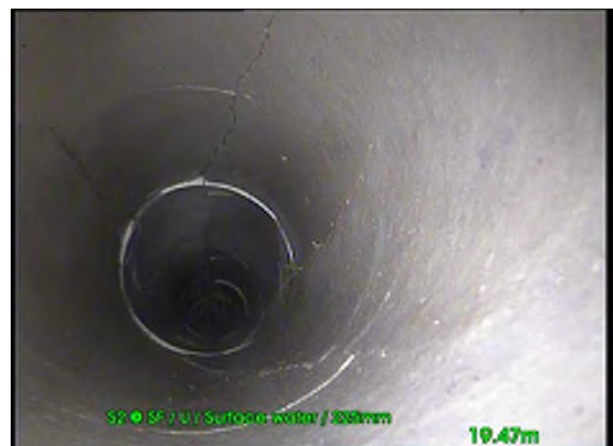
Photo: 43_43_545_A.jpg, 00:01:53 19.47m, Fracture, multiple, from 12 to 12 o'clock, Start
