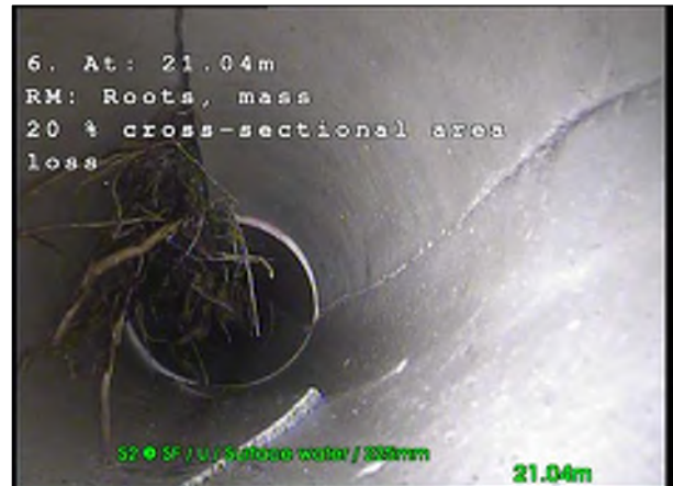
Photo: 43_43_376_A.jpg, 00:02:07 21.04m, Roots, mass, 20% cross-sectional area loss, Start
