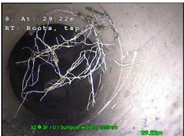
Photo: 43_43_378_A.jpg, 00:02:58 29.22m, Roots, tap
