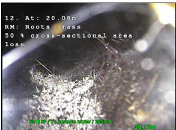
Photo: 37_37_303_A.jpg, 00:01:59 20.08m, Roots, mass 50 % cross-sectional area loss
