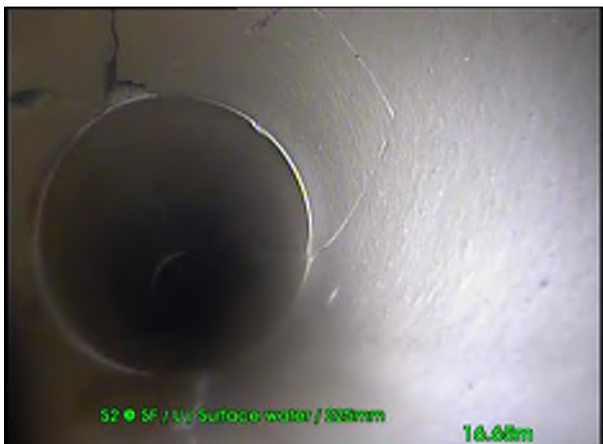
Photo: 44_44_556_A.jpg, 00:02:06 16.65m, Hole in drain/sewer, at 11 o'clock
