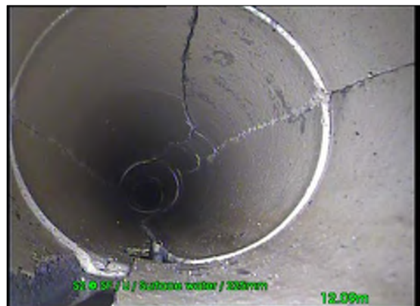
Photo: 42_42_534_A.jpg, 00:01:44 12.09m, Hole in drain/sewer, at 7 o'clock
