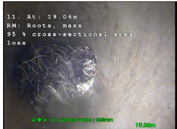
Photo: 38_38_317_A.jpg, 00:02:23 19.06m, Roots, mass 95 % cross-sectional area loss
