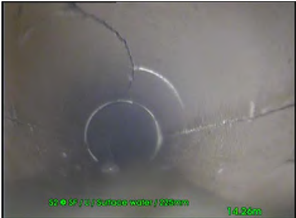
Photo: 38_38_310_A.jpg, 00:00:14 3.11m, Fracture, multiple, from 12 to 12 o'clock, Start
