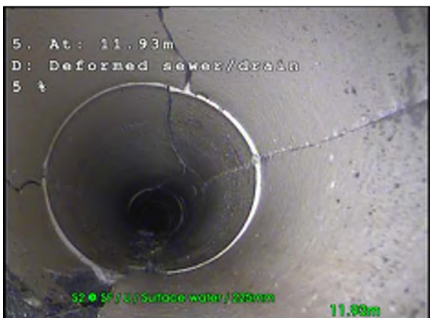
Photo: 43_43_375_A.jpg, 00:01:15 11.93m, Deformed sewer/drain 5 %
