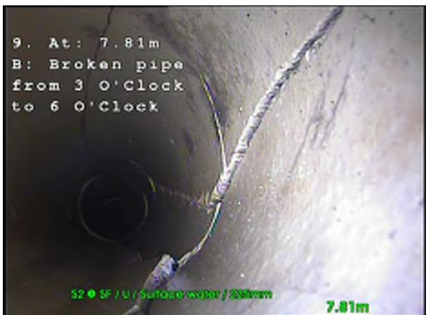
Photo: 42_42_354_A.jpg, 00:01:12 7.81m, Broken pipe from 3 O'Clock to 6 O'Clock
