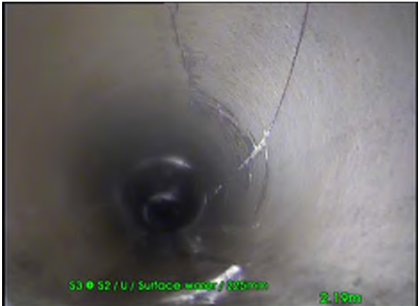
Photo: 47_47_578_A.jpg, 00:00:12 1.45m, Fracture, multiple, from 12 to 12 o'clock, Start
