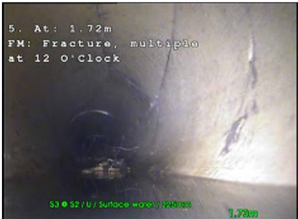
Photo: 46_46_405_A.jpg, 00:00:17 1.72m, Fracture, multiple, from 12 to 12 o'clock, Start
