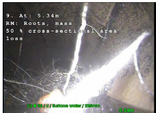
Photo: 46_46_409_A.jpg, 00:00:38 5.34m, Roots, mass 50 % cross-sectional area loss
