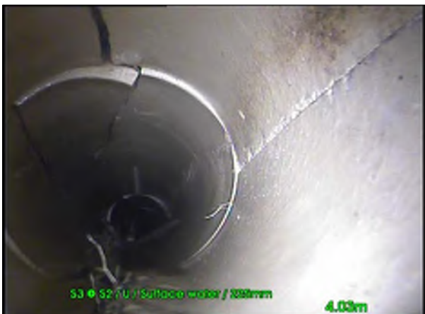
Photo: 47_47_580_A.jpg, 00:00:39 4.03m, Deformed sewer/drain, 10%
