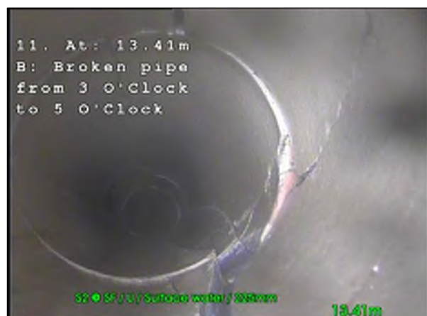
Photo: 41_41_340_A.jpg, 00:02:14 13.41m, Broken pipe from 3 O'Clock to 5 O'Clock
