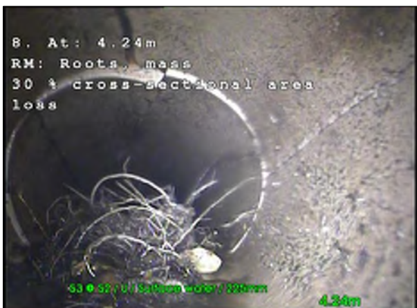
Photo: 46_46_408_A.jpg, 00:00:32 4.24m, Roots, mass 30 % cross-sectional area loss
