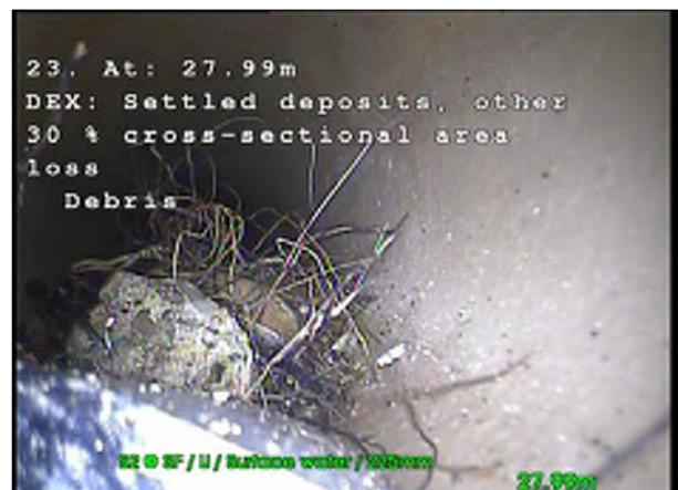
Photo: 42_42_368_A.jpg, 00:04:27 27.99m, Settled deposits, other 30 % cross-sectional area loss Debris
