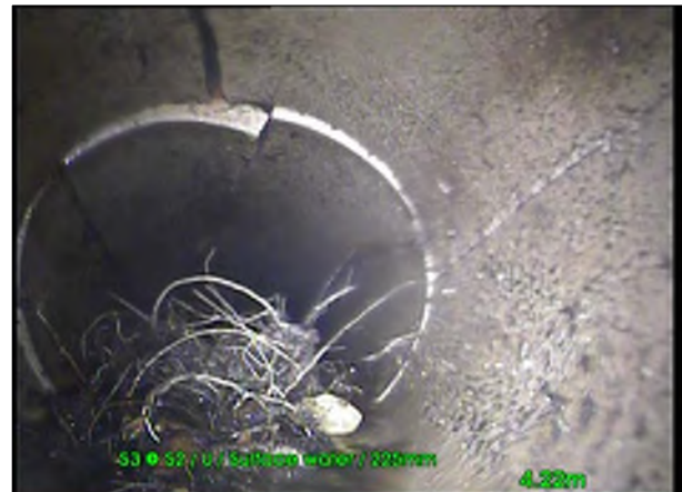
Photo: 46_46_407_A.jpg, 00:00:30 4.24m, Broken pipe from 9 O'Clock to 12 O'Clock
