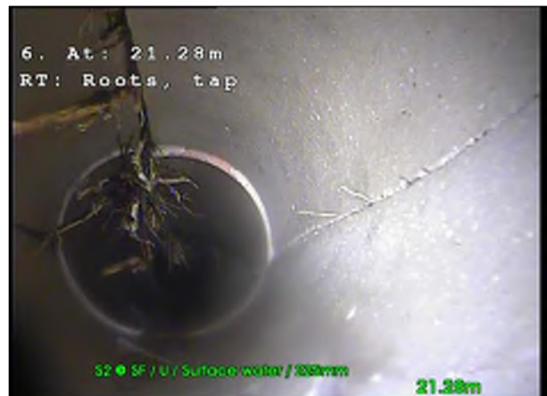
Photo: 44_44_564_A.jpg, 00:02:38 21.28m, Roots, tap
