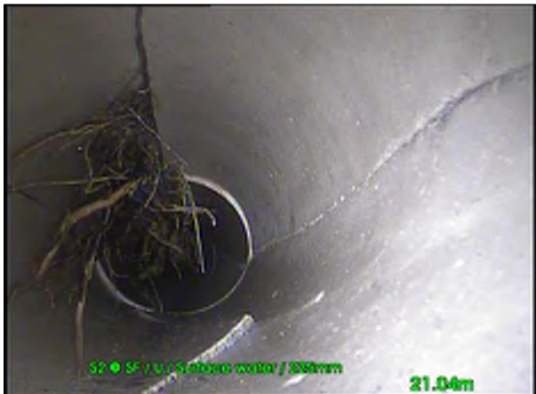
Photo: 43_43_546_A.jpg, 00:01:59 20.1m, Broken pipe, from 12 to 12 o'clock, Start
