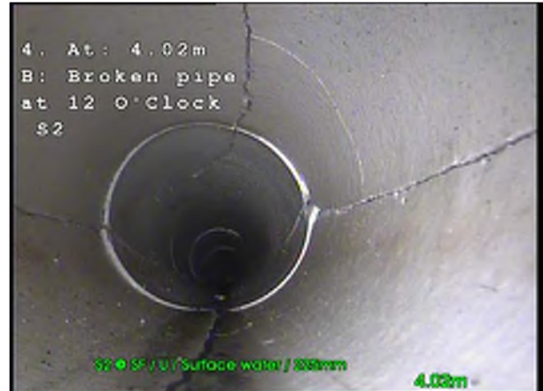
Photo: 43_43_542_A.jpg, 00:00:30 4.02m, Broken pipe, from 12 to 12 o'clock, Start
