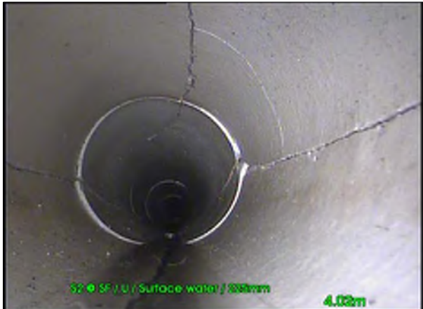
Photo: 43_43_540_A.jpg, 00:00:20 2.44m, Fracture, multiple, from 12 to 12 o'clock, Start
