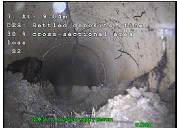
Photo: 37_37_298_A.jpg, 00:00:56 9.04m, Settled deposits, fine 30 % cross-sectional area loss S2
