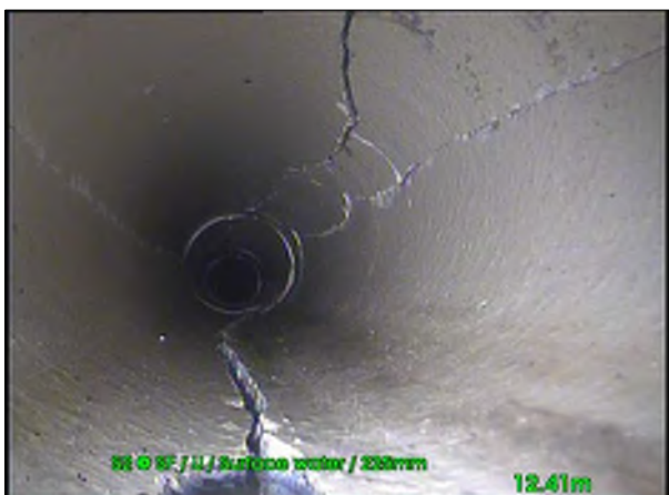
Photo: 42_42_535_A.jpg, 00:01:46 12.41m, Hole in drain/sewer, at 6 o'clock
