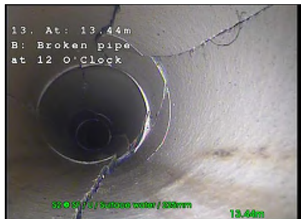
Photo: 42_42_358_A.jpg, 00:02:07 13.44m, Broken pipe, from 12 to 2 o'clock
