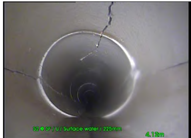
Photo: 44_44_555_A.jpg, 00:00:41 4.12m, Broken pipe, from 12 to 12 o'clock, Start
