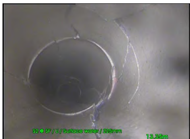
Photo: 41_41_526_A.jpg, 00:01:59 13.35m, Deformed sewer/drain, 5%
