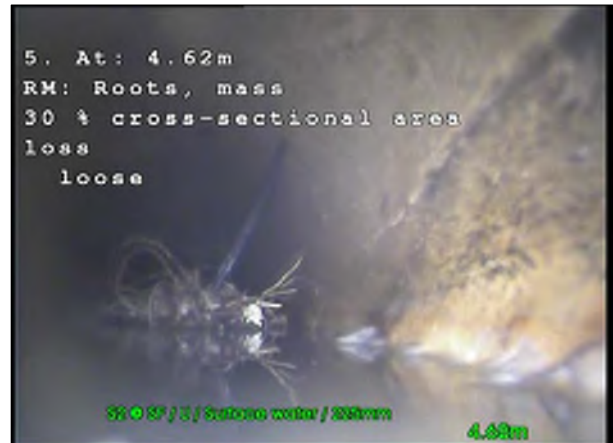
Photo: 39_39_323_A.jpg, 00:00:24 4.62m, Roots, mass 30 % cross-sectional area loss loose
