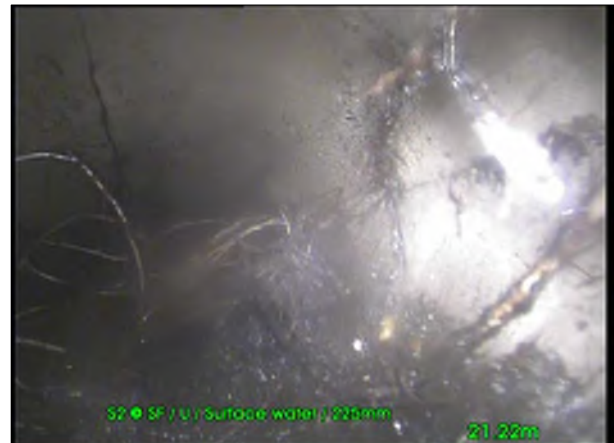
Photo: 41_41_528_A.jpg, 00:03:35 21.22m, Roots, mass, 35% cross-sectional area loss
