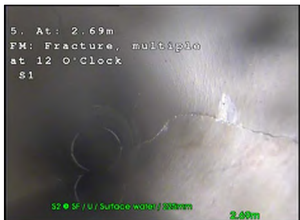
Photo: 41_41_334_A.jpg, 00:00:28 2.69m, Fracture, multiple, from 12 to 12 o'clock, Start
