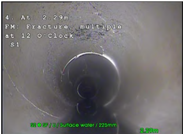
Photo: 44_44_553_A.jpg, 00:00:32 2.29m, Fracture, multiple, from 12 to 12 o'clock
