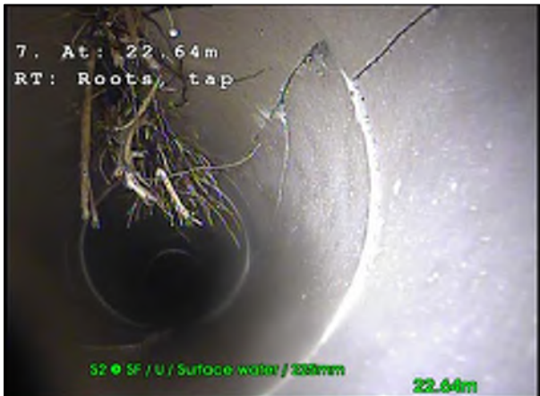
Photo: 44_44_386_A.jpg, 00:03:04 22.64m, Roots, tap
