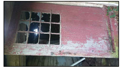
3. Yard doors to be preserved and re located in front of the original position
