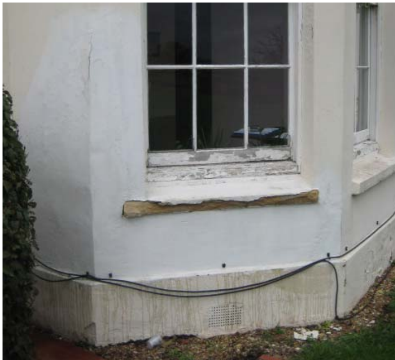
Detail of the existing outside sills to be repaired
