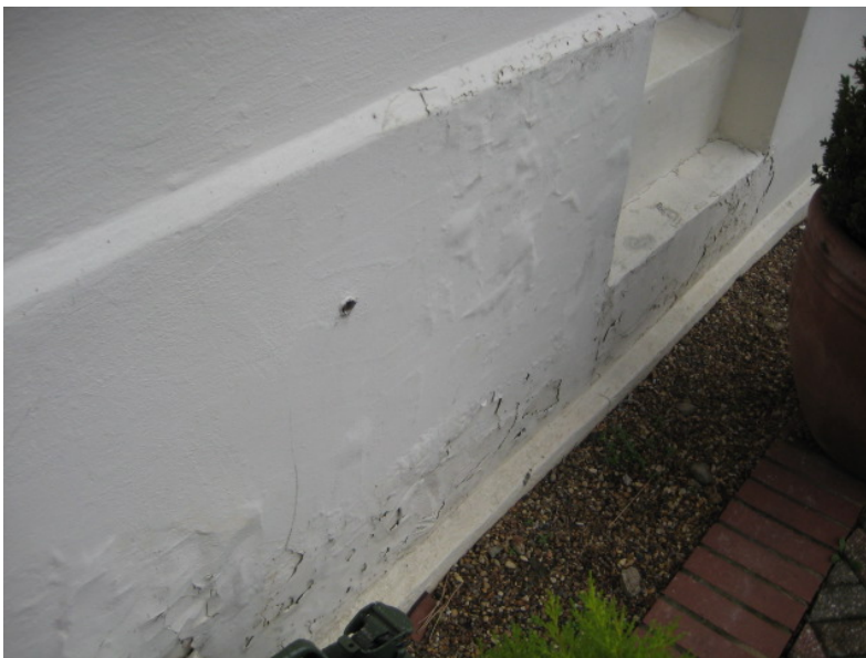
Detail of the existing plaster damaged by the humidity
