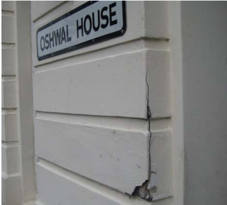
Detail of the existing plaster damaged by cracks
