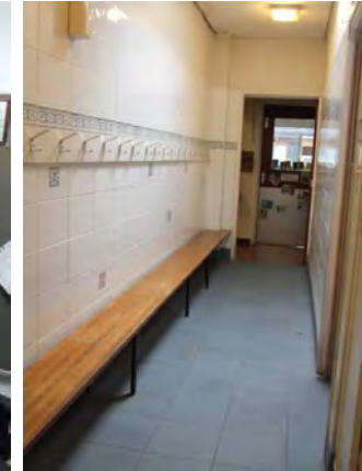
An existing corridor is also used as the boys changing area. When in use access to parts of the school are restricted.
