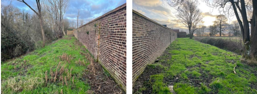
Figures 2 and 3: Views (outside the walled garden) of the southern wall where two new openings are proposed
