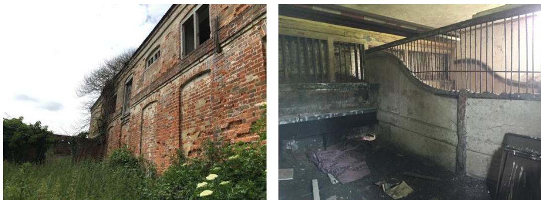
Figures 15 and 16: Close up view of the stable's east elevation (left) and interior view (right) (photographs taken c.2017)
