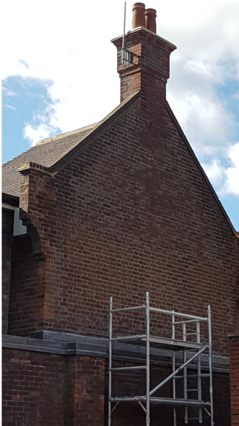
Rear elevation showing inset of common bricks following works (After Brick Treatment)
