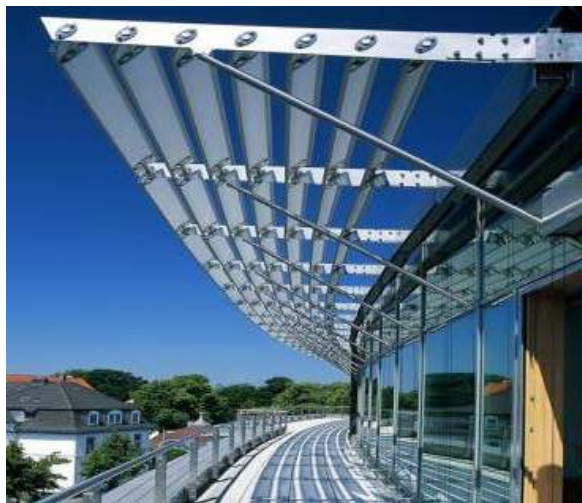
Solar PV Louvres on the South Facade
