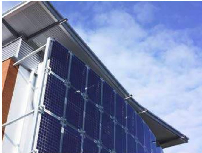
Photovoltaic Installations: Project Epic (BREEAM Excellent Office)
