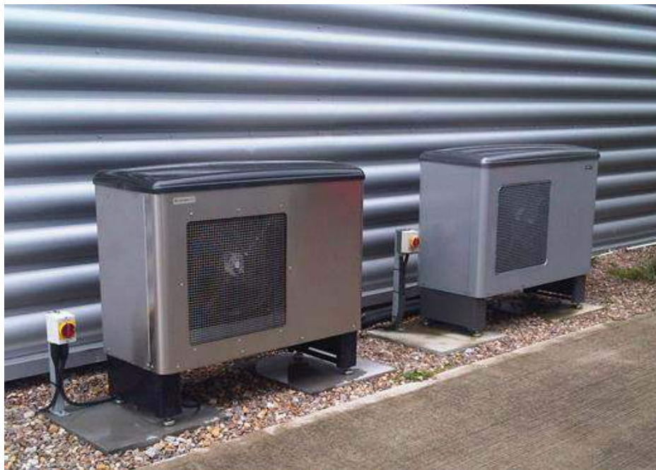
Air Source Heat Pumps
