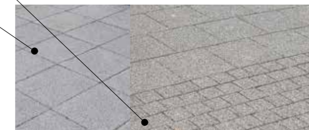
Concrete slab/ block paving in natural/ grey
