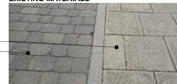
Rumbled effect Block paving. Service Road. Slab paving in natural colours. Pedestrian footpath
