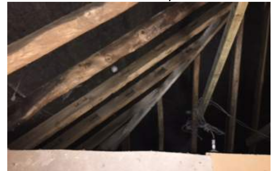
Distressed timber rafters to roof of unit 1
