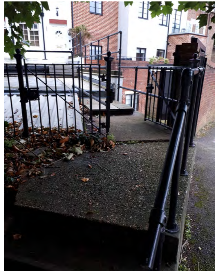
Access to the flats 33a, 34a from the rear pavement, off Batterdale
