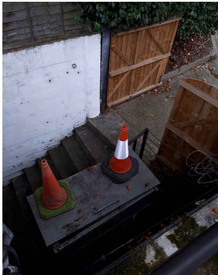
Stairs providing access to the service yard from the rear of the property
