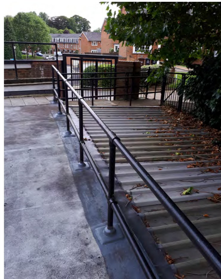
View over terrace to the rear looking toward Batterdale, showing temporary cover over service yard below with protective railings providing guarding
