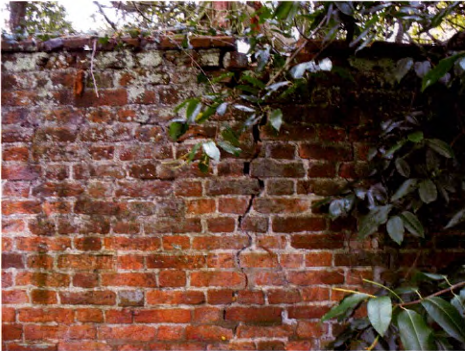
Ph 5 : Detail of South Wall showing condition
