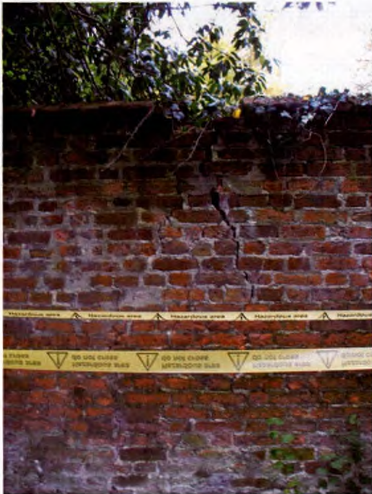
Ph 6 : Detail of East Wall showing condition
