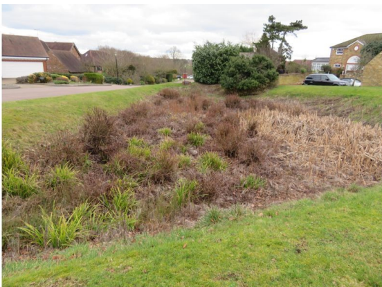
7 - Pond 4, virtually dry attenuation pond choked by vegetation.
