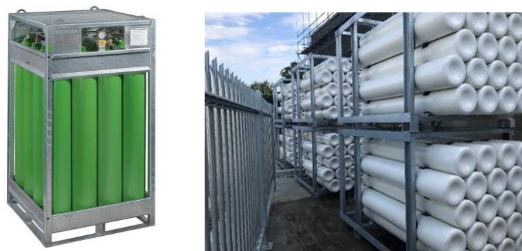
Figure 3.2.3. – CNG Storage Cylinder Packs
