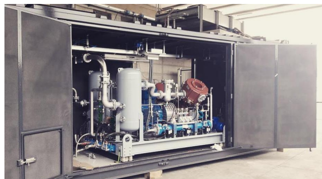
Figure 3.2.2. – Inside main section of Compressor Housing showing Compressor
