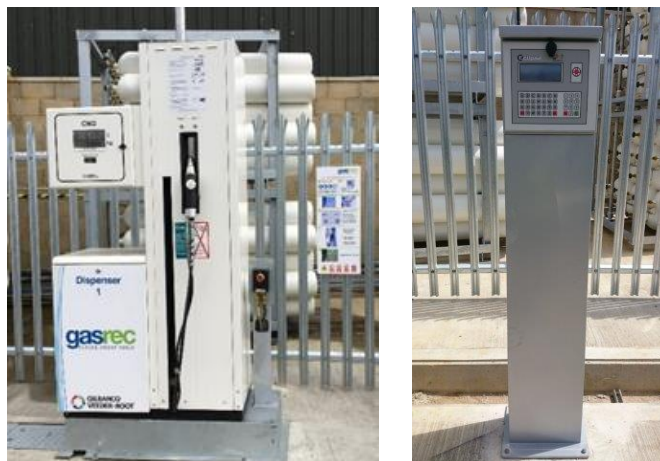
Figure 3.2.4. – CNG Dispenser and Fuel Management Unit
