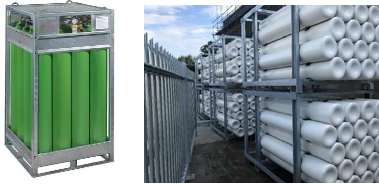
Figure 1.5.2 – CNG Storage Cylinder Racks
