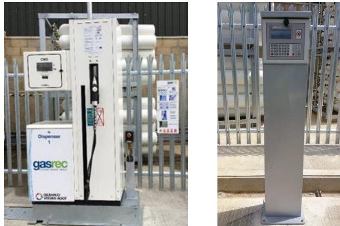
Figure 1.5.3 – CNG Dispenser and Fuel Management Unit
