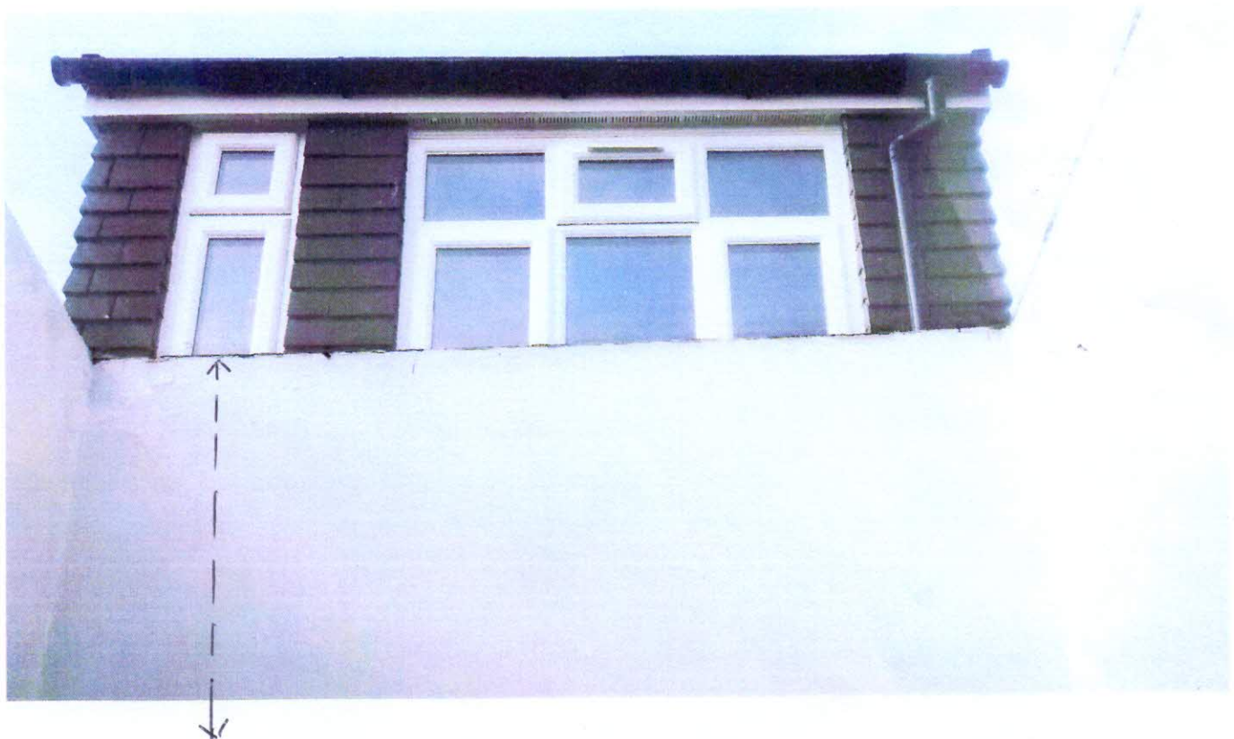
UNAUTHORISED 4 th DORMER WINDOW LOOKING INTO NO 43 BEDROOM SKYLIGHT
