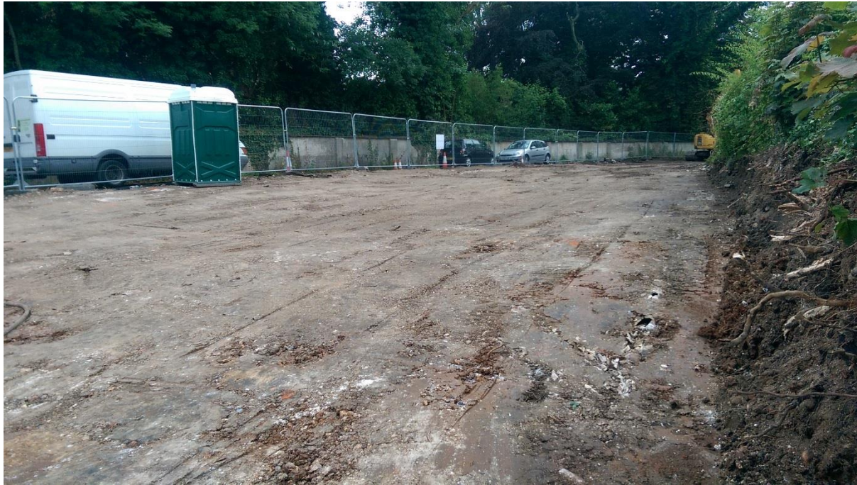
Photographs 3 & 4 - The photographs above and below show some views of the site once all of the soil containing Japanese knotweed has been removed and the areas have been backfilled.
