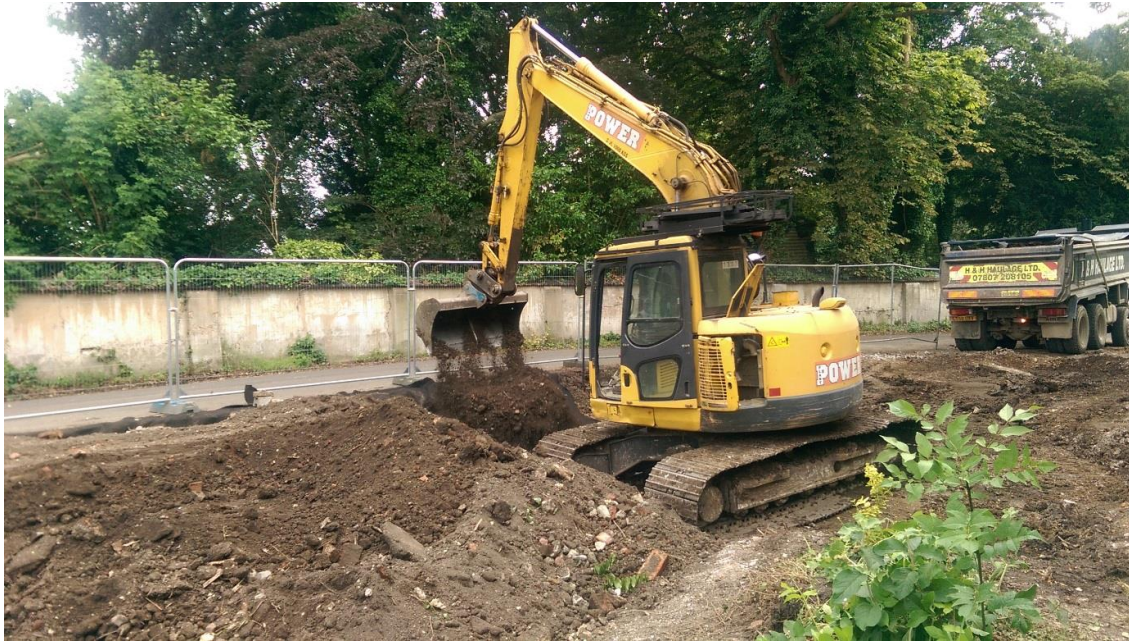
Photographs 1 & 2 – These photos show an area of the affected site being excavated by TP Knotweed Solutions Ltd.
