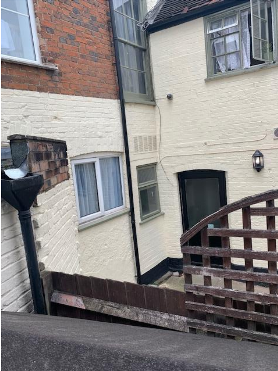
Photograph above: The rear ground floor (west) window of No. 44 (to the left of the rainwater down pipe), which faces into the rear courtyard of The Eight Bells PH. The line of the downpipe indicates the division between the two buildings.
