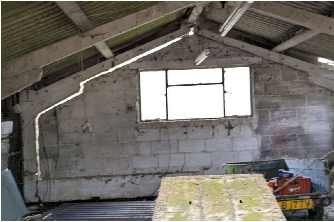
Photograph 5 View on rear elevation showing separation of infill blockwork and precast frame.
