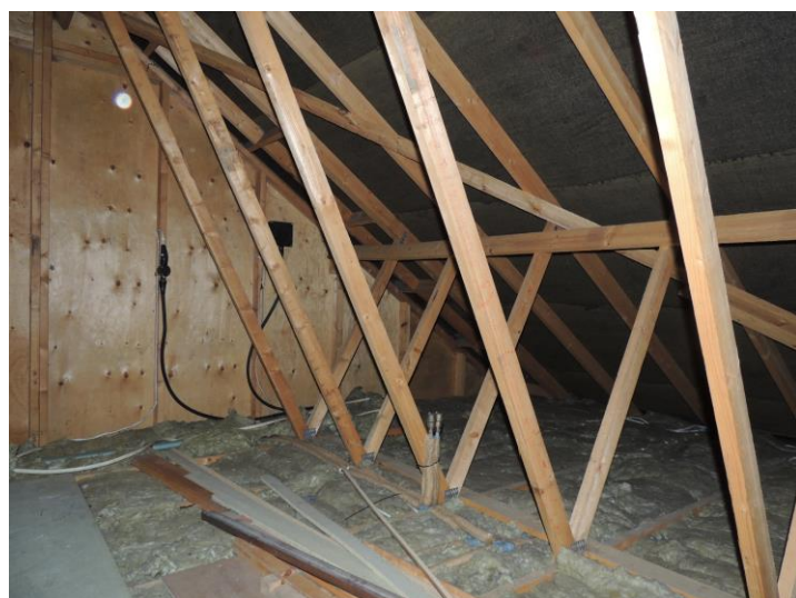
Photo 7: Note cluttered roof and lack of evidence of bats on floor of loft
