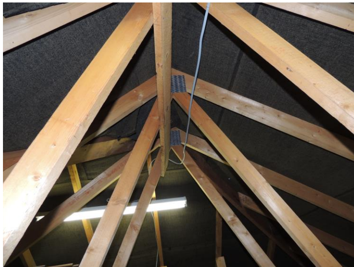
Photo 14: Note lack of conventional ridge board
