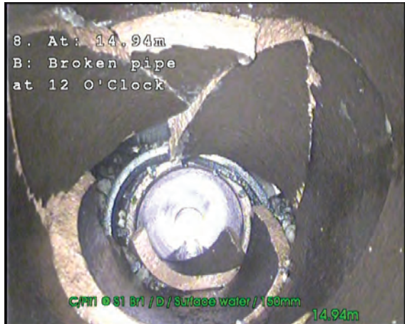
Photo: 6_6_31_A.jpg, 00:01:28 14.94m, Broken pipe, from 12 O'Clock to 12 O'Clock
