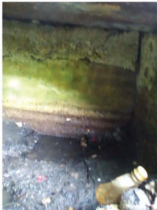
Image B:- View of outfall from ditch under concrete entrance
