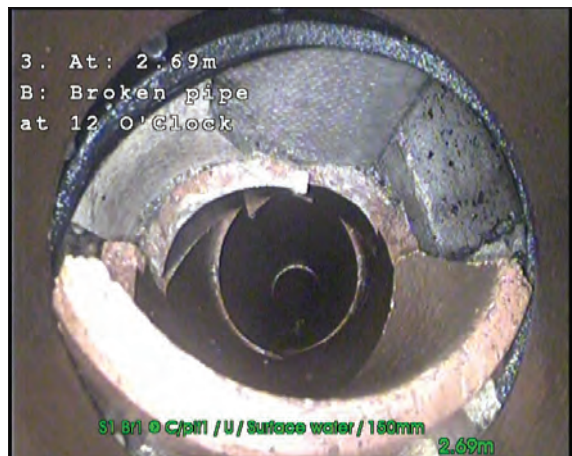
Photo: 5_5_22_A.jpg, 00:00:26 2.69m, Broken pipe, from 12 O'Clock to 12 O'Clock
