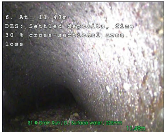
Photo: 2_2_7_A.jpg, 00:01:12 11.49m, Settled deposits, fine 30 % cross-sectional area loss (removed)
