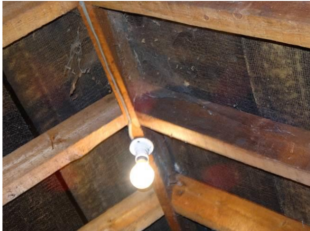
Photograph 18: Beams with cobwebs containing moth wings.
