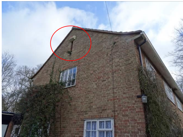
Photograph 15: Building with hole in the gable end of the roof allowing access into the loft space (circled in red).
