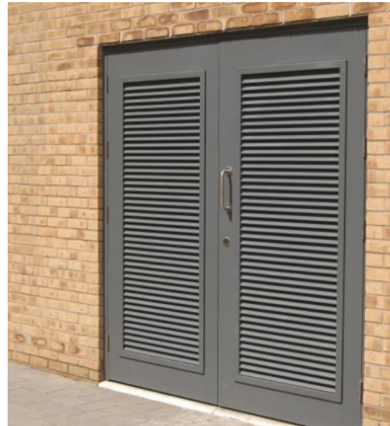
Substation / bin store / cycle store Grey Aluminium Louvred Door Colour: Grey RAL 7031
