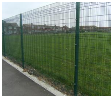
Image 15; Typical paladin boundary security fencing polyester powder coated steel – colour RAL 6005 – green
