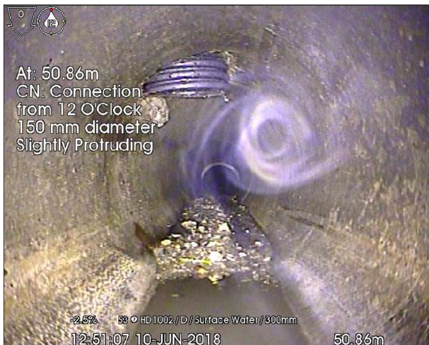
Photo: 1 - S3 downstream to HD1002_50-86m_125107.jpg 50.86m, CN: Connection from 12 O'Clock 150 mm diameter Slightly Protruding
