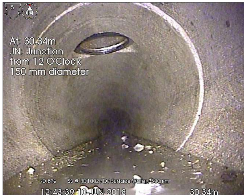
Photo: 1 - S3 downstream to HD1002_30-34m_124339.jpg 30.34m, JN: Junction from 12 O'Clock 150 mm diameter
