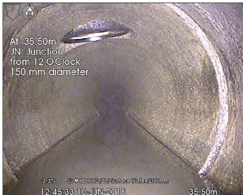
Photo: 1 - S3 downstream to HD1002_35-50m_124533.jpg 35.5m, JN: Junction from 12 O'Clock 150 mm diameter
