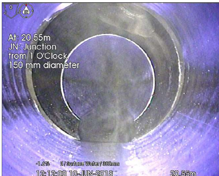
Photo: 2 - S3 upstream to S4_20-55m_121200.jpg 20.55m, JN: Junction from 1 O'Clock 150 mm diameter
