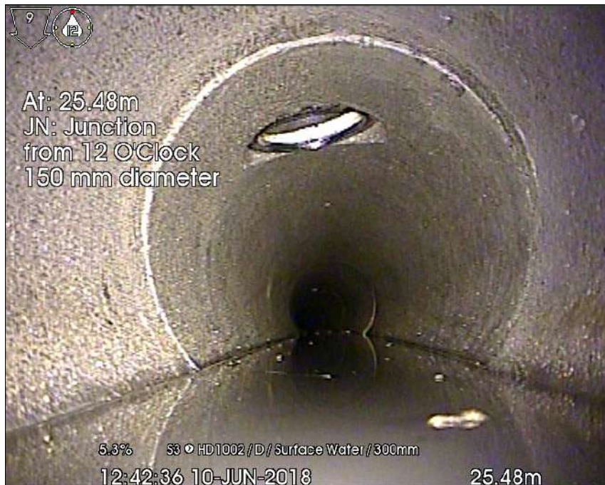
Photo: 1 - S3 downstream to HD1002_25-48m_124236.jpg 25.48m, JN: Junction from 12 O'Clock 150 mm diameter
