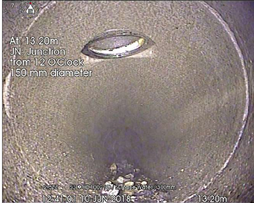
Photo: 1 - S3 downstream to HD1002_13-20m_124101.jpg 13.2m, JN: Junction from 12 O'Clock 150 mm diameter
