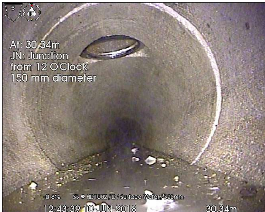
Photo: 1 - S3 downstream to HD1002_30-34m_124339.jpg 30.34m, JN: Junction from 12 O'Clock 150 mm diameter
