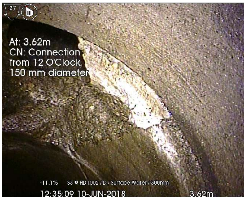
Photo: 1 - S3 downstream to HD1002_3-62m_123509.jpg 3.62m, CN: Connection from 12 O'Clock 150 mm diameter
