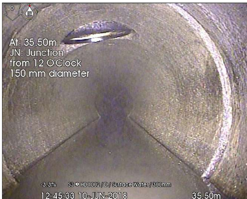
Photo: 1 - S3 downstream to HD1002_35-50m_124533.jpg 35.5m, JN: Junction from 12 O'Clock 150 mm diameter
