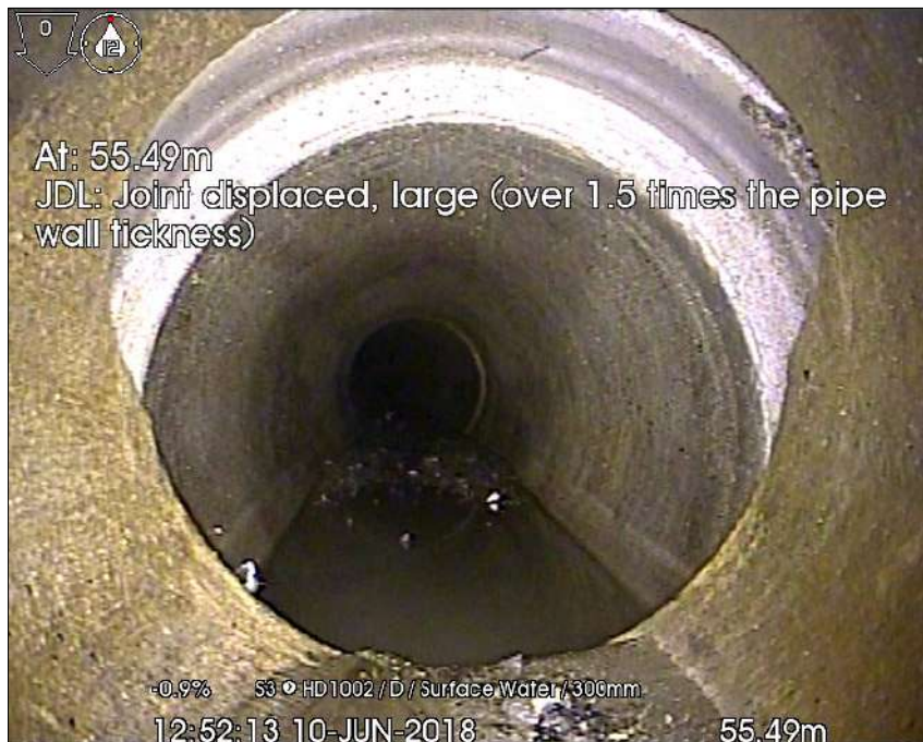
Photo: 1 - S3 downstream to HD1002_55-49m_125213.jpg 55.49m, JDL: Joint displaced, large (over 1.5 times the pipe wall tickness)
