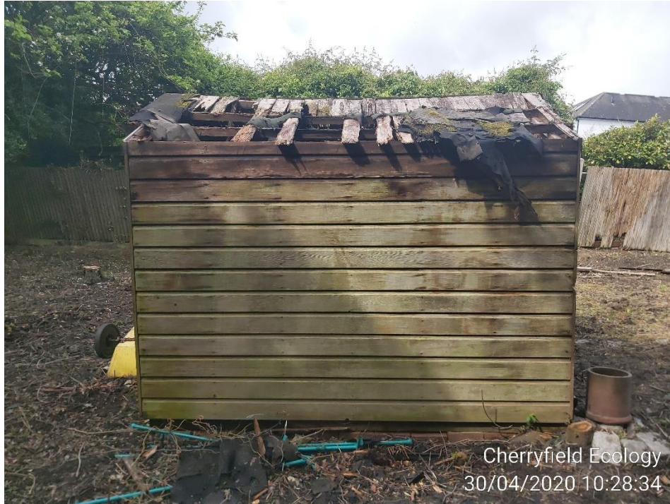
Figure 4: Side elevation and damaged roof
