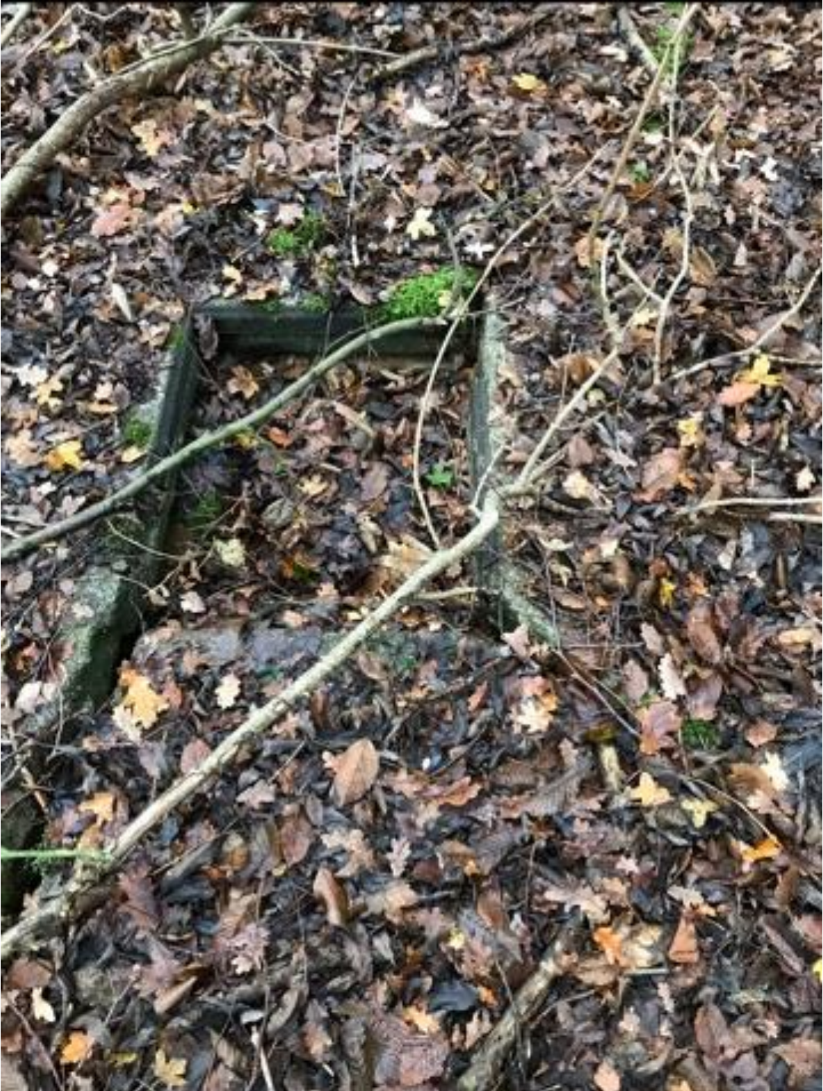
Figure 4: Evidence of drainage left from the demolition of Hook Cottages
