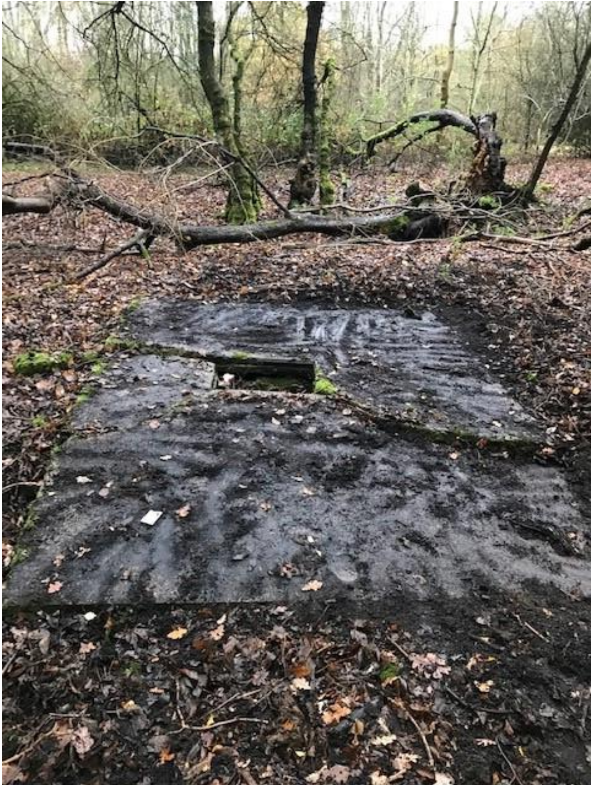
Figure 5: Evidence of drainage left from the demolition of Hook Cottages
