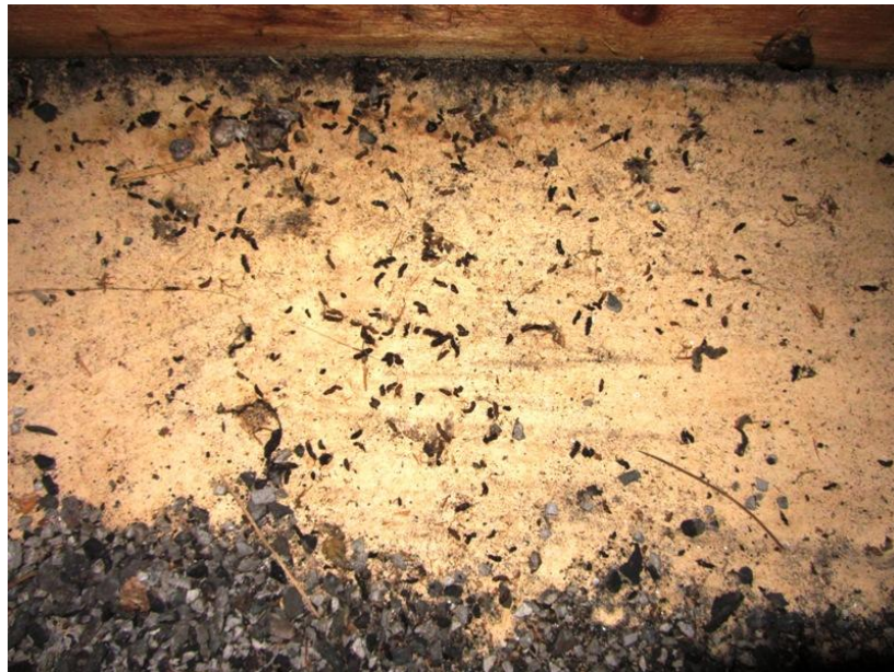
Photograph 8 : Example of bat droppings in loft void
