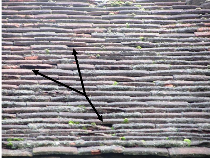
Photograph 7 : Example of raised tiles on rear elevation
