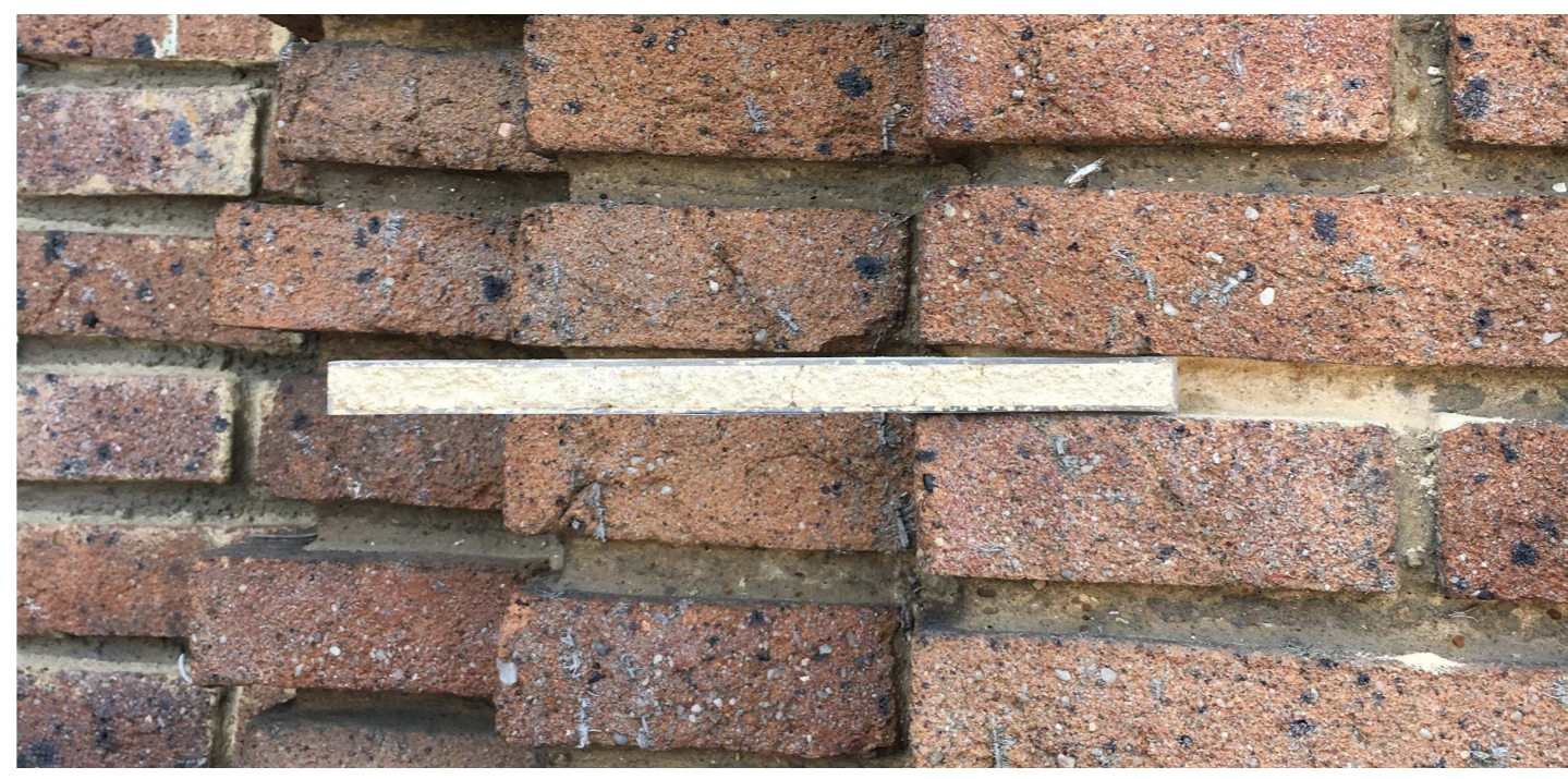
Proposed Heritage mortar (to match existing) shown on the existing Heritage brickwork Mortar reference Ecoright 'Grosvenor'
