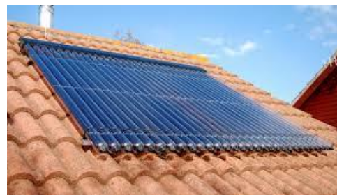
Figure 6 – Solar Thermal Panels
