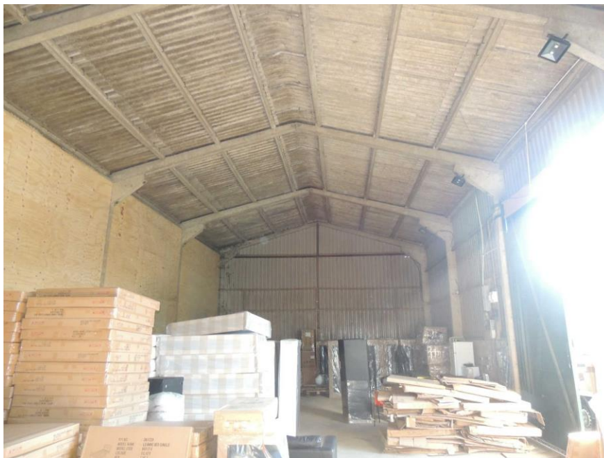
Photo 5: Looking north-eastwards in Building 2. Note lack of features that might be occupied by bats
