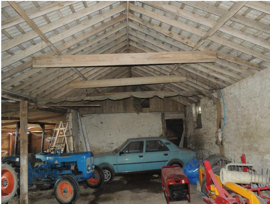
Photo 16: Looking south-westwards along the single-storey brick barn. Note lack of features that might be occupied by bats
