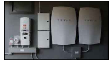
TESLA POWERWALL 2 AC BATTERY PACK MAX OUTPUT 7 Kw EXCESS TO MAINS or GRID 1150H X 755W X 155D INC pv INVERTER
