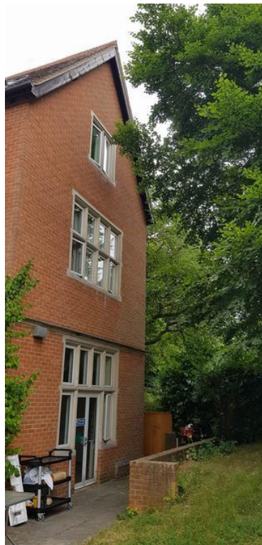
Image 16 T288 close to the building, recommended to be cut back to clear the building by 2-3m
