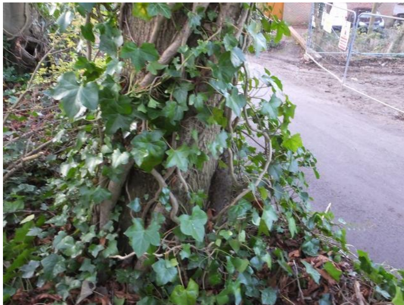
Image 12 T274, growing over the top of the retaining wall
