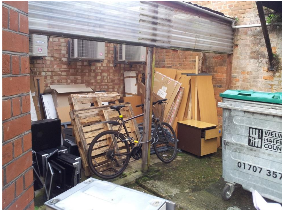
The space between the listed buildings is currently used for storing refuse and is in need of the kind of environmental improvements that the proposals would bring.
