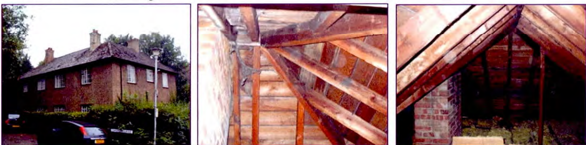
Left – right: Eastern and northern elevations of the building; loft interior of number 23 Church Lane.
