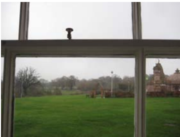
Bespoke design for doors and windows to match the existing windows (Sample for the outlook of the material).
