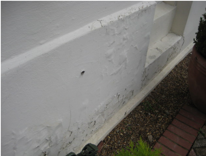
detail of the existing plaster damaged by water ingress
