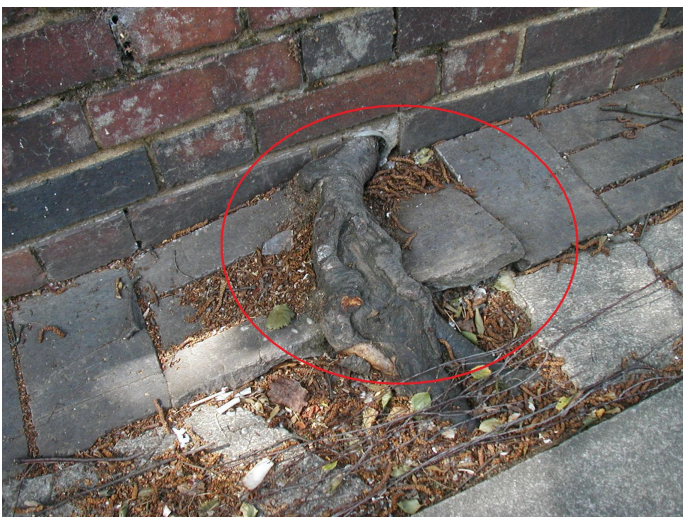
5/ Damage Caused by Roots of T19
