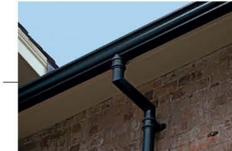
BLACK UPVC GUTTERS AND DOWNPIPES
