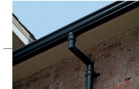
BLACK upvc GUTTERS AND DOWNPIPES
