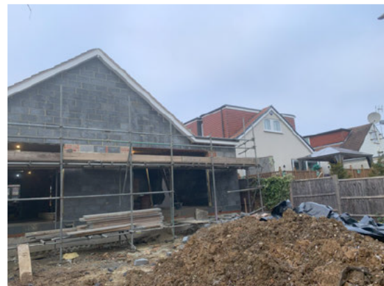
View of the rear of 21 Theobalds Road and the dormers to roof of 19 and 17 Theobalds Road.
