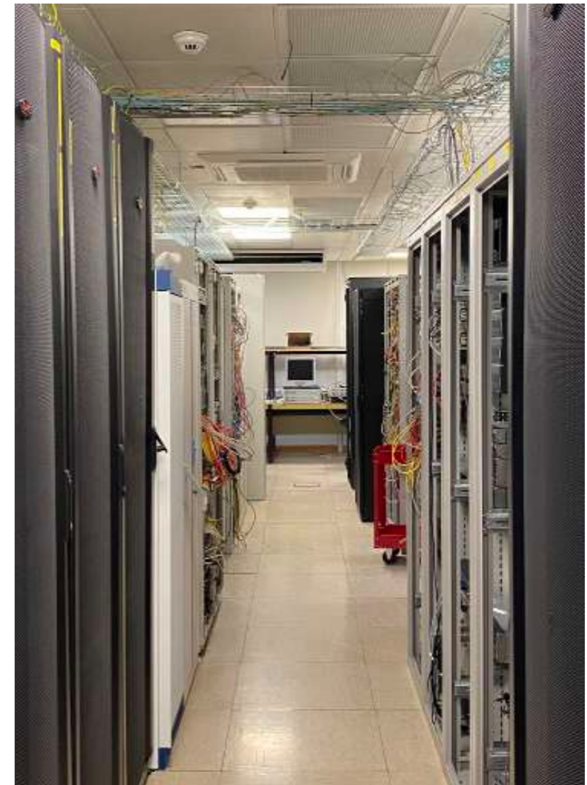
Figure 1.3 : An example of existing of Inmarsat's equipment racks arrangement / positioning.
