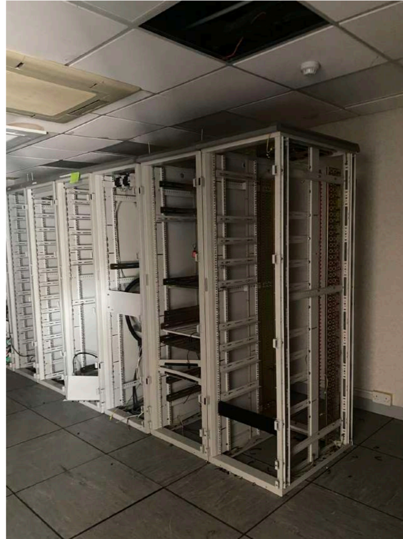
Figure 1.2 : Example of equipment racks
