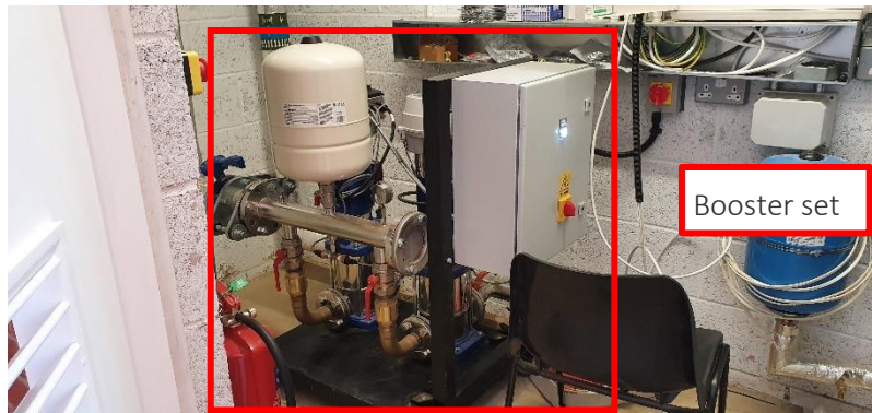
Figure 2-3 Water booster set
